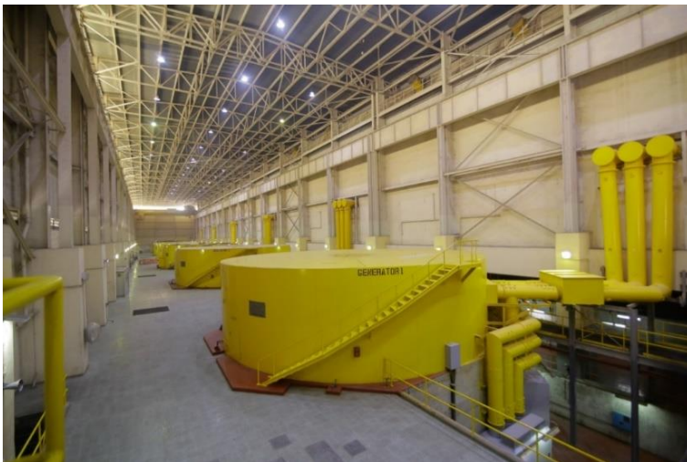
Figure 6: Generating unit Jebba Hydropower plant
