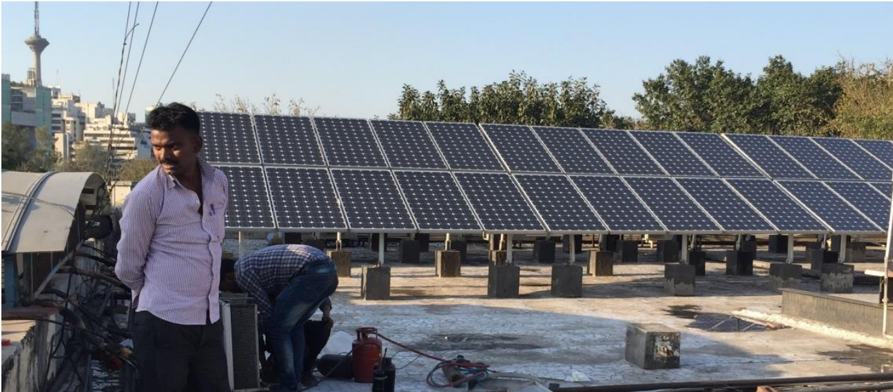
Figure 7: Rooftop Solar in India
