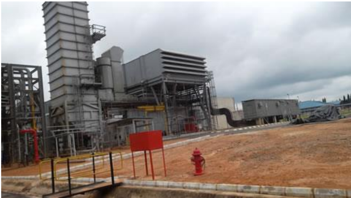
Aba Geometric power plant. Source: geometricpower.com
